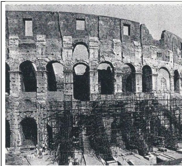
Figure 7b. Support of the arcades: the seven masonry pillars [4]. Reinforcement of pillars with steel and Epoxy resin injections through holes
