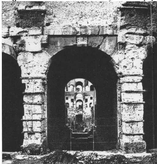
Figure 7a. The pillars #18 and #19 before restoration and after the travertine cladding has been taken away.
