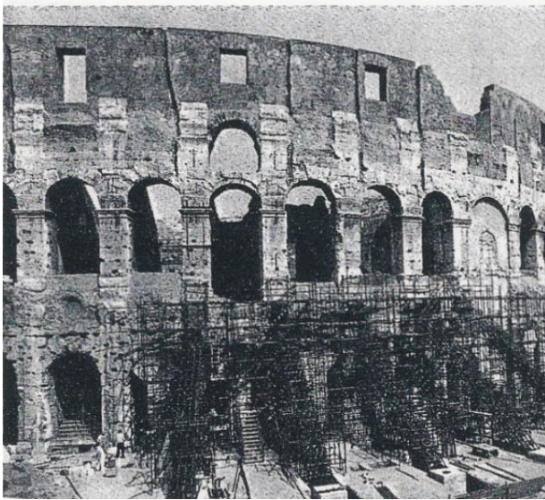
Figure 5b. Support of the arcades. Reinforcement of n. 6 pillars with steel and Epoxy resin injections through holes
