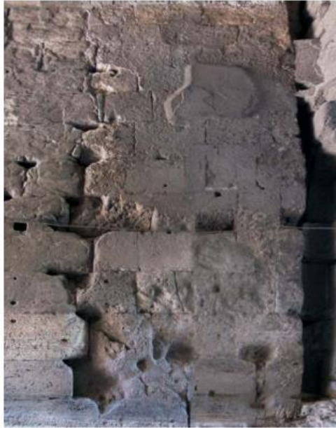
Figure 9. Pillar # 49, left, 1st level, disconnections 10 irregular and 11 regulars.
